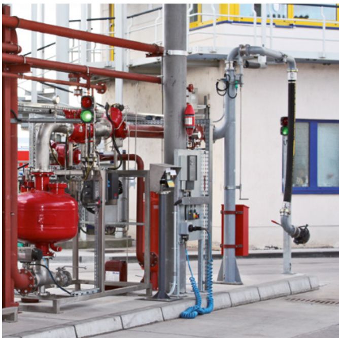
↓ CMS: compact metering skid
