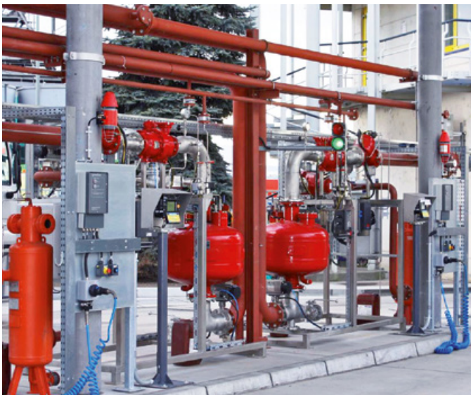
↑ CMS: compact metering skid
